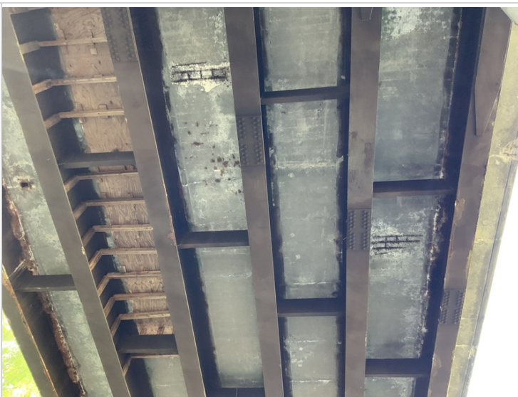
Spalls Span 1 bays 1 and 3
