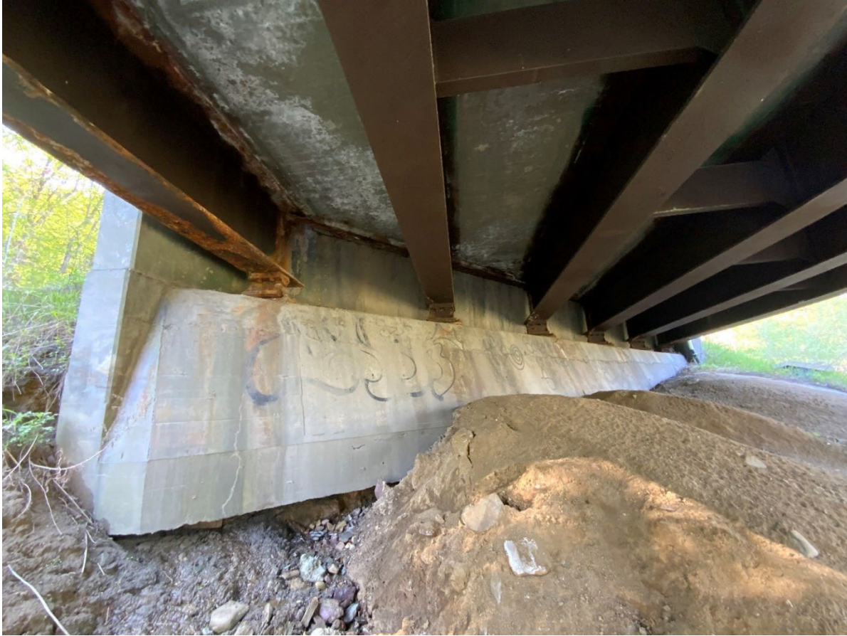
Appendix A 2: Abutment 1. Note some undermining of the left side of the abutment.
