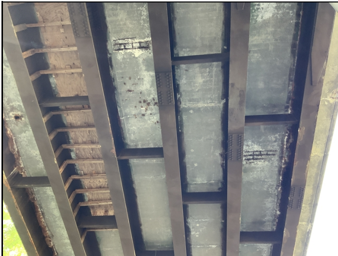
Spalls Span 1 bays 1 and 3
