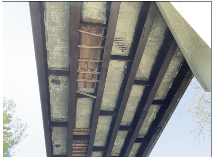
Spall span 2 bay 3
