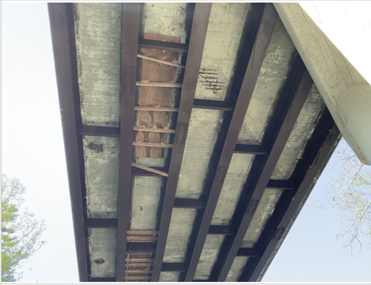
Spall span 2 bay 3
